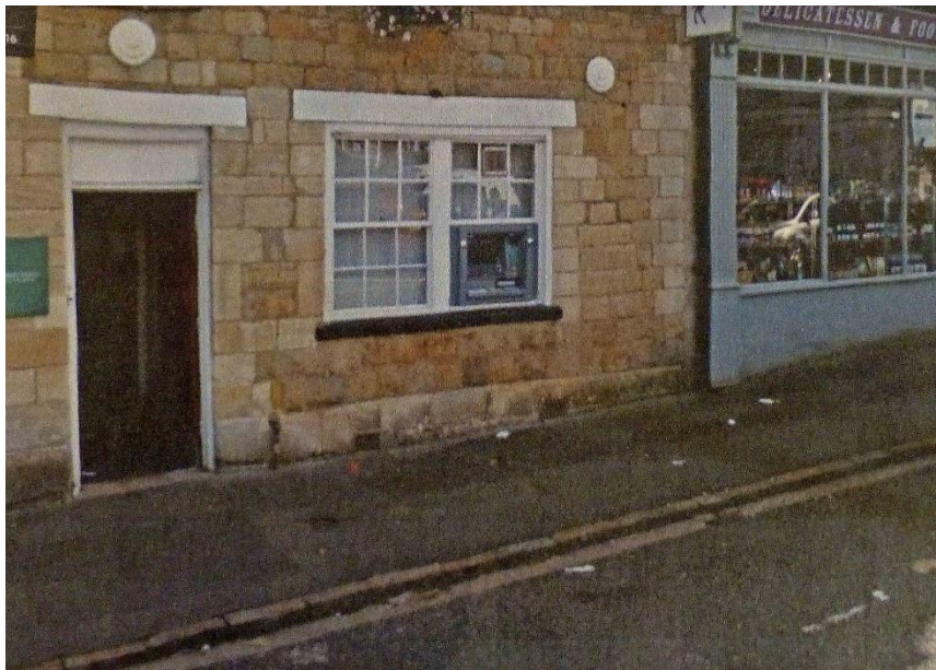
Photo 1: Patchwork of tarmac within the pavements on the High Street
